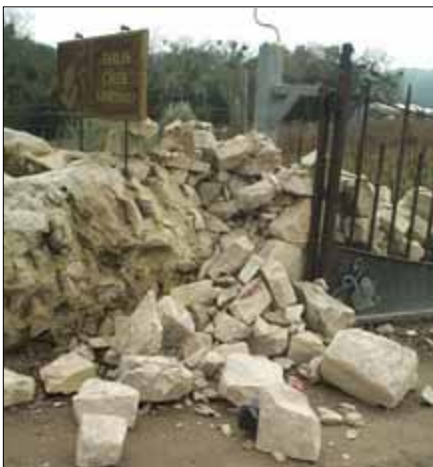
The front gate was one of the casualties of the December 22 earthquake.
